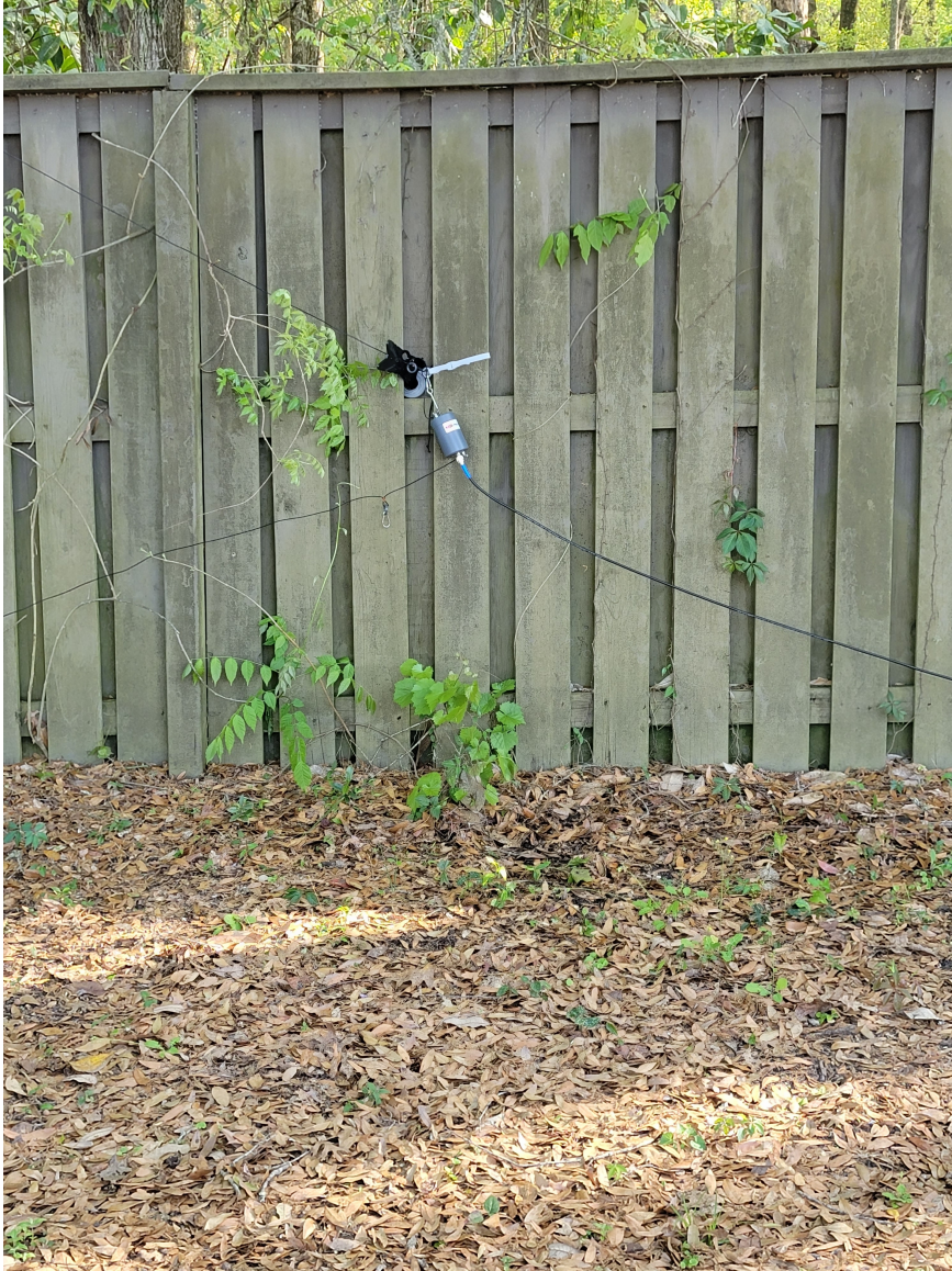
Ad Hoc antenna switch to allow Alachua County EOC to choose between antennas on the fly.
