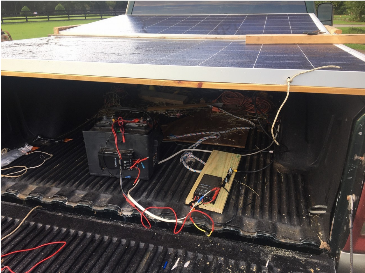
Solar Panel setup from 2020; in 2021 we used only 1 panel.
