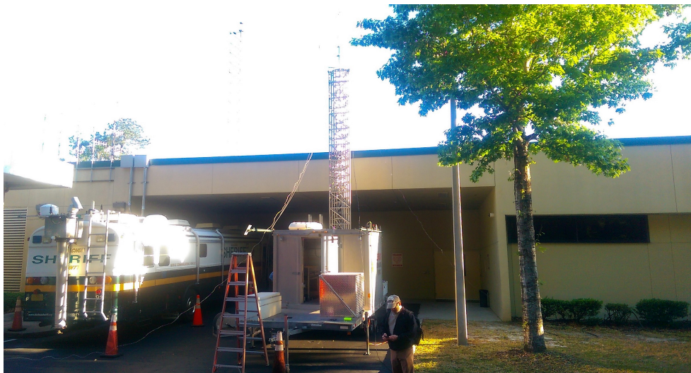
Mobile antenna tower getting ready to deploy at the EOC
